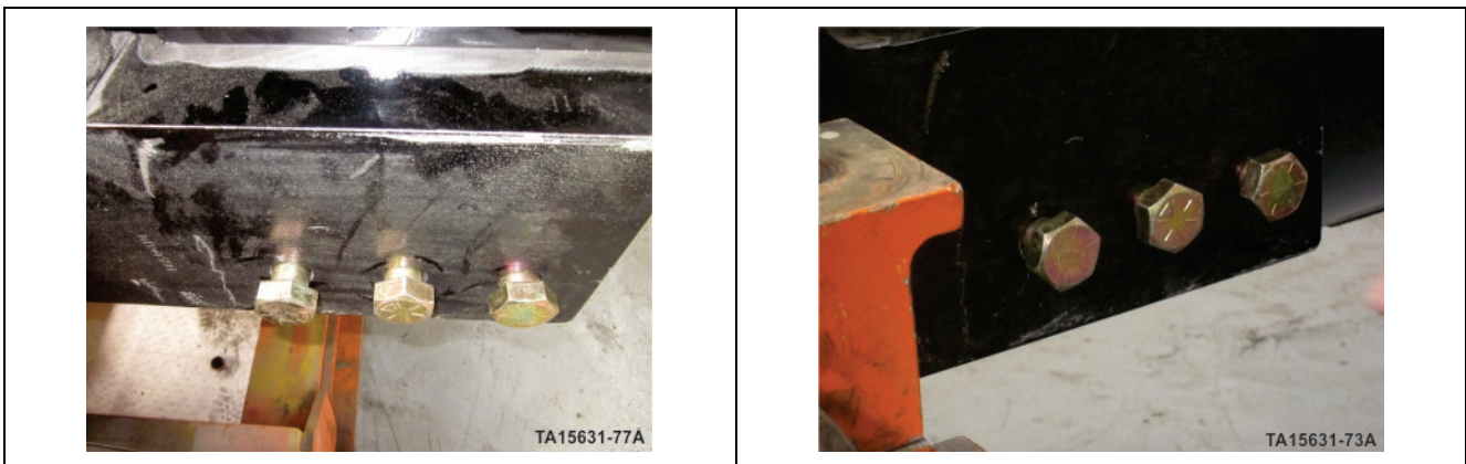
Figure 89. Generators with horizontally installed bolts in mounting feet
