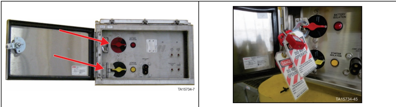
Battery Isolation Box – Battery isolation switch in OFF position with locks in place
