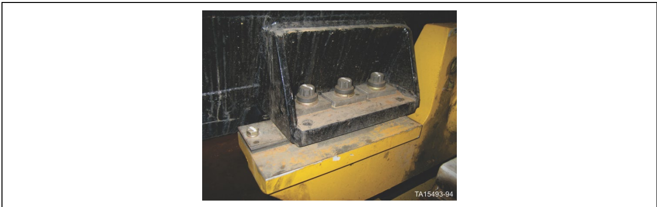
Figure 88. Generators with vertically installed bolts in mounting feet
